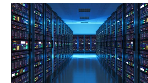
CF Borden Data Center
